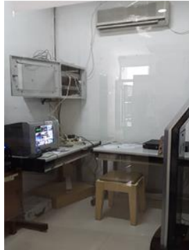
Gambar. 5.20. Ruang Kontrol Panel
