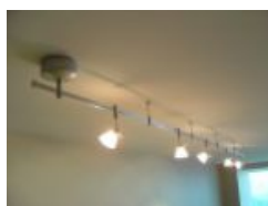
Gambar 2.27. Track Lighting System
